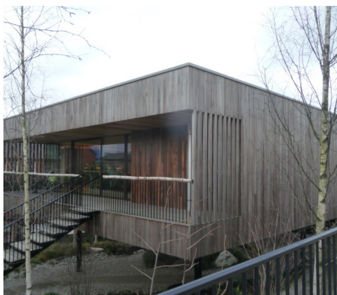
U.S. tulipwood cladding at Maggie’s Centre, Oldham, one year after it’s opening.
